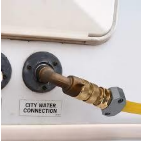
Fill line to non-portable tank with a quick disconnect coupler
